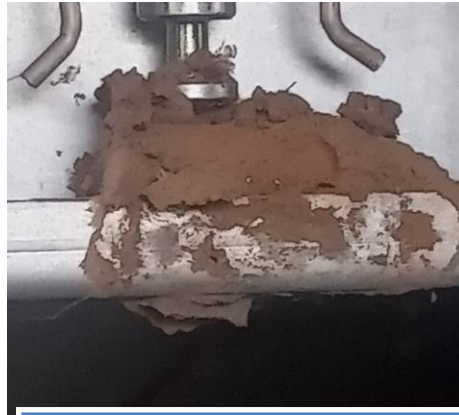
Ant nest built inside the 11kV panel
