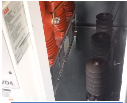
11kV Breaker and Surge arrester compartment after maintenance,
