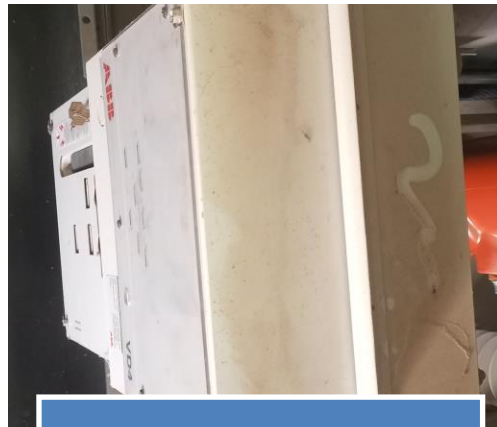
Rear part of panel covered with dust
