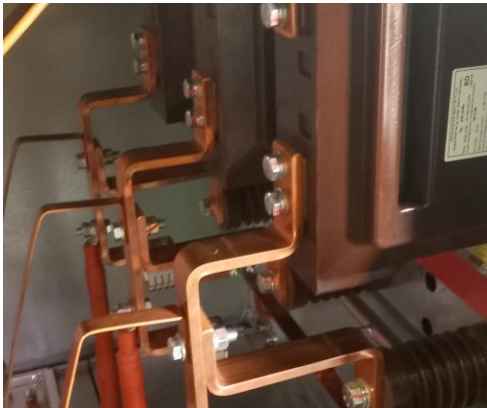
CT after maintenance.
