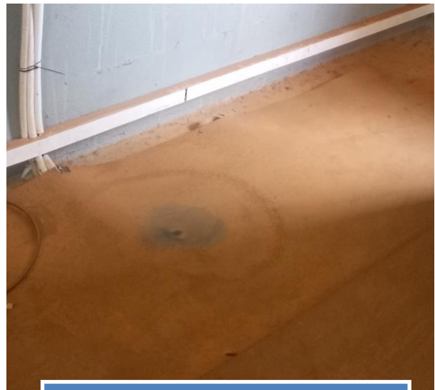
Thick choking dust behind the panels..
