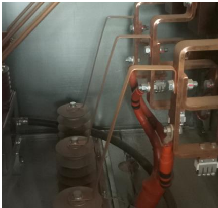
Heavy Dusty Switchgear panel
