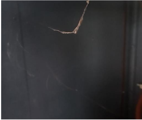
Interior panel covered with in cobwebs.
