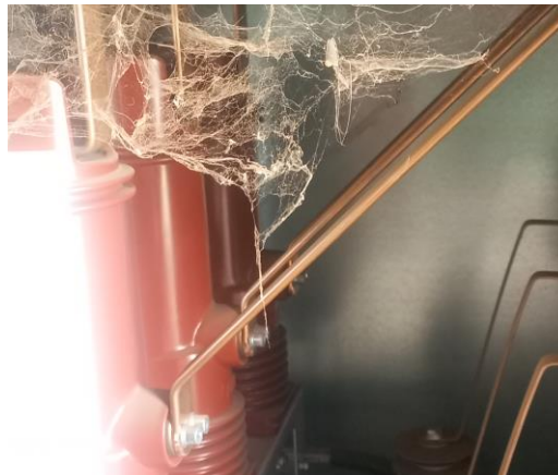
Thick cobwebs with small droplets of water seen inside the panel which can be a source of serious arc flash..
