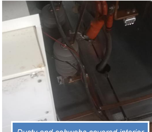
Dusty and cobwebs covered interior part of the 11kV panel
