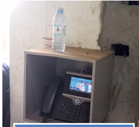
Telephone receiver covered in dangerously thick dust.
