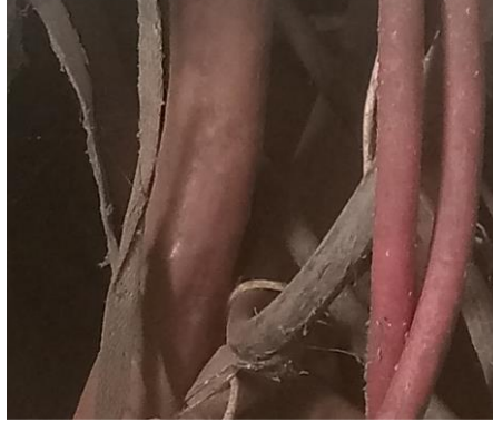
The dusty cable trench that goes up the panel through the cable openings to the panels.
