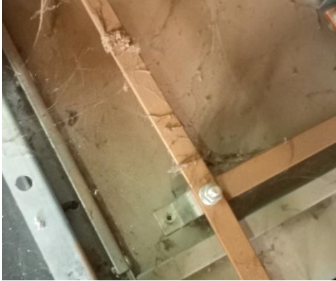
Panel Earth bars covered in dust and cobwebs.
