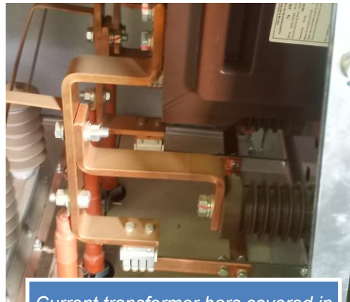
Current transformer bars covered in dust.
