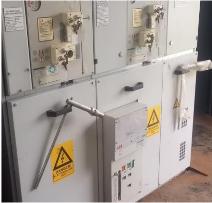
External dusty panel and floor before maintenance
