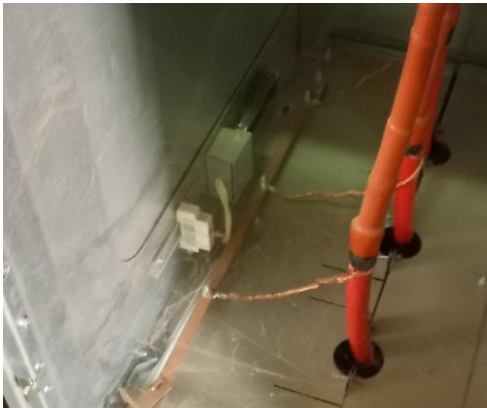
Open halls from cable trench to 11kV panel power cable compartment.
