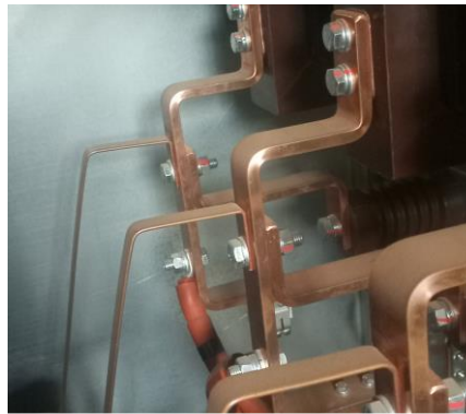
Dusty Switchgear interior parts
