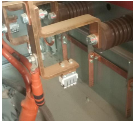
Dusty porcelain Insulators and the panel floor
