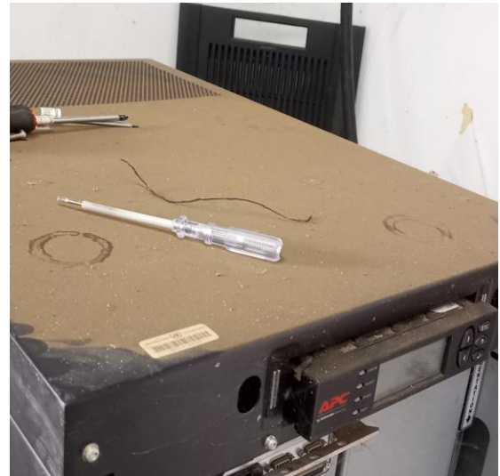
UPS covered with thick dust which destroyed it.
