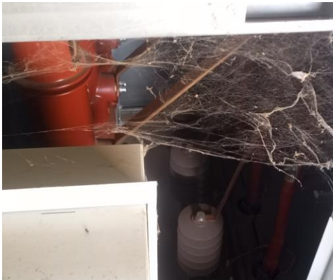
Interior panel fully covered with cobwebs and dust.
