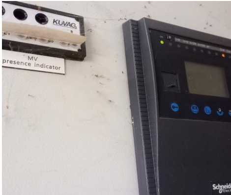
Schneider relay covered in cobwebs.
