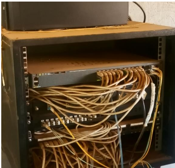
Communication switch covered in thick dust
