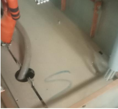
Open through passage from the cable trench to the panel which invites reptiles in the panel because of the warmth
