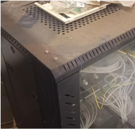
Communication switch covered in thick dust
