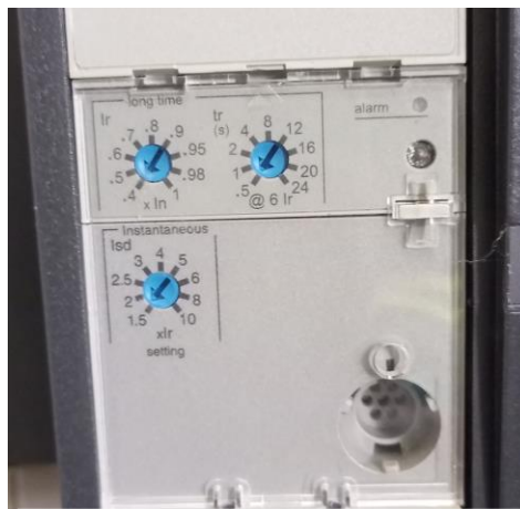
MCCB setting point on MCCB.
