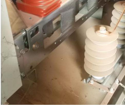
Surge arrester compartment covered in dust and cobwebs.
