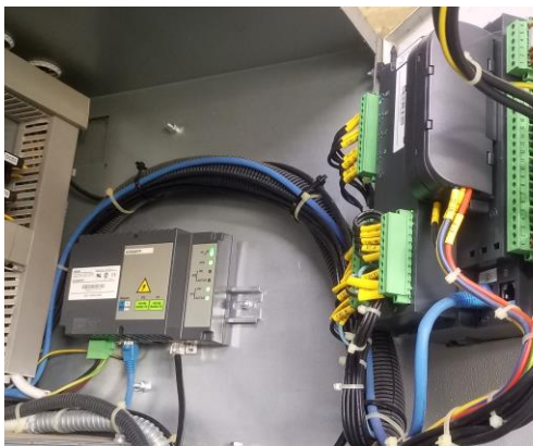
Internal control wiring and relay after maintenance
