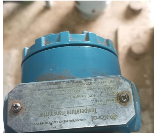
Transformer temperature transducer to Protection relay not configured or wired..
