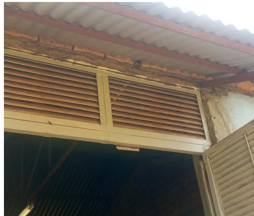
Non covered ventilations with dust from outside flowing inside..
