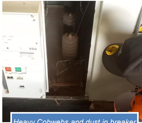
Heavy Cobwebs and dust in breaker compartments.
