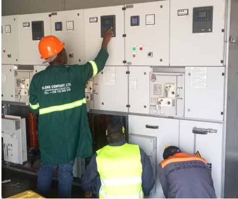
Overcurrent test being prepared.
