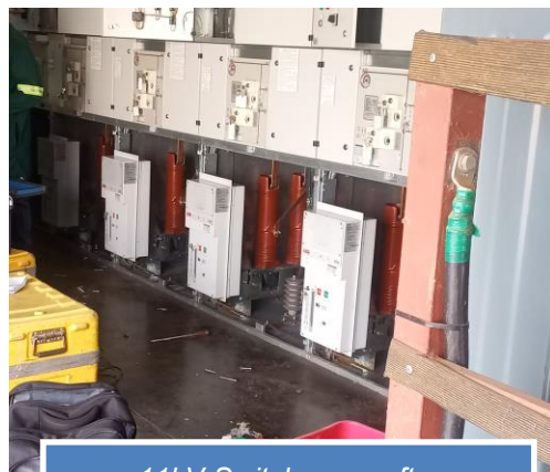
11kV Switchgears after maintenance.
