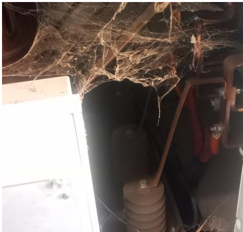
Thick Cobwebs and dust inside the panel
