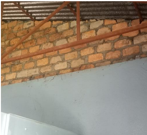
Lack of cement plastered roof with dust falling to the floor as lizards move along the wall.
