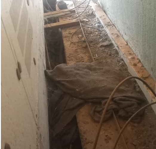
Cable trench with old blanket covered in very thick dust.
