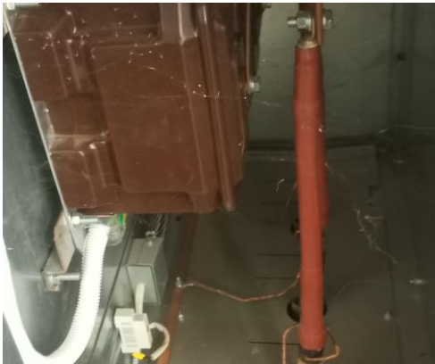
Cobwebs covering current transformer compartments
