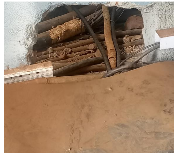
S03 plant house with open chisel wall to the outside with a danger of snakes entrance and habitation.
