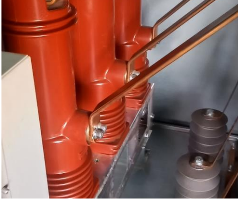
11KV compartment after maintenance
