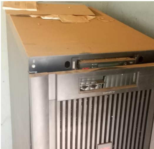
UPS in a very sorry dust soaked state.
